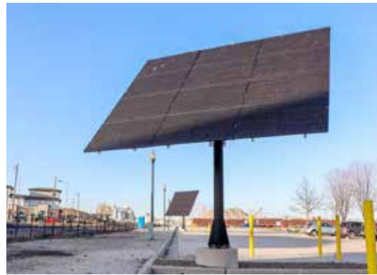
Solar panel installed at Leicht Park. Photo credit: City of Green Bay Public Works Planning
